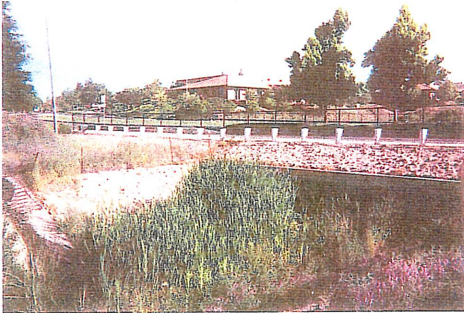
Plate 13 – Linda Creek below Rocky Ridge Drive. The aquatic vegetation below this box culvert should only be cleared when the integrity of the culvert and/or concrete embankments are in jeopardy. The remaining vegetation would typically lie down during flood events and would not inhibit flow movement.
